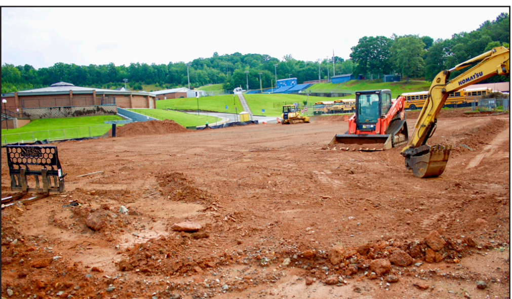
The site of the Towns County Schools Agricultural Facility will look remarkably different by January 2025, which is when Superintendent Dr. Darren Berrong hopes construction will be finished. Photo by Lowell Nicholson
